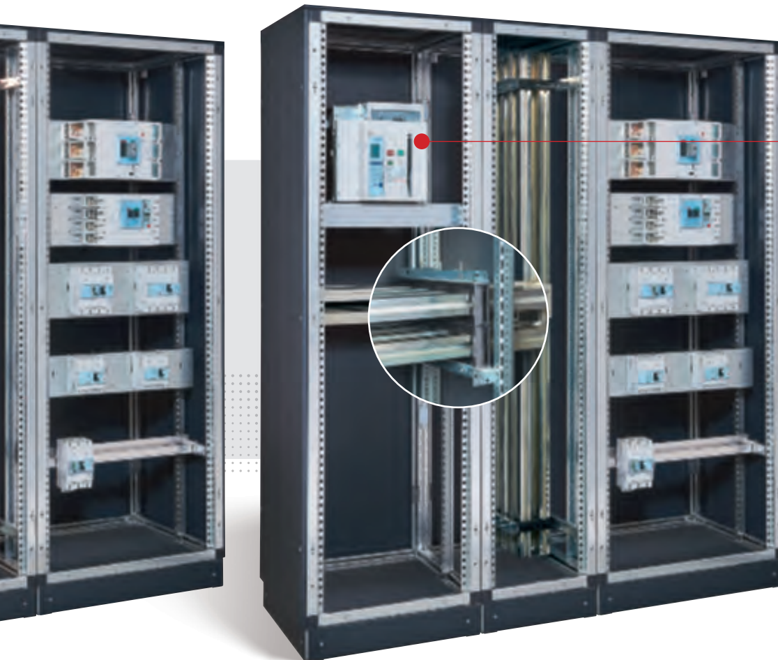
XL 3 S 4000 equipped with C-section aluminium busbars Mounted vertically at the side in cable sleeve + transfer horizontal
